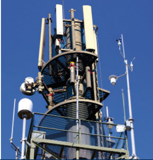
Cell Tower Distribution Box
